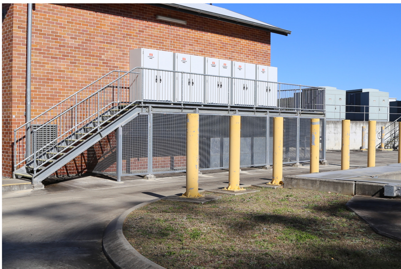
Lower Wyong Pump Station
